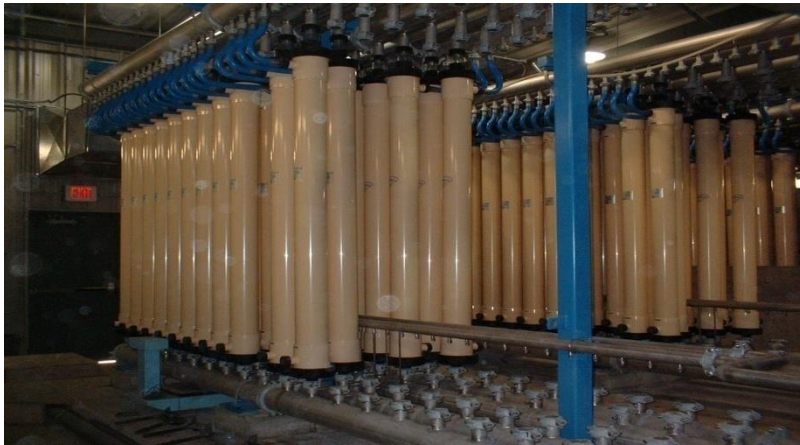
Microfiltration water plant, USA
