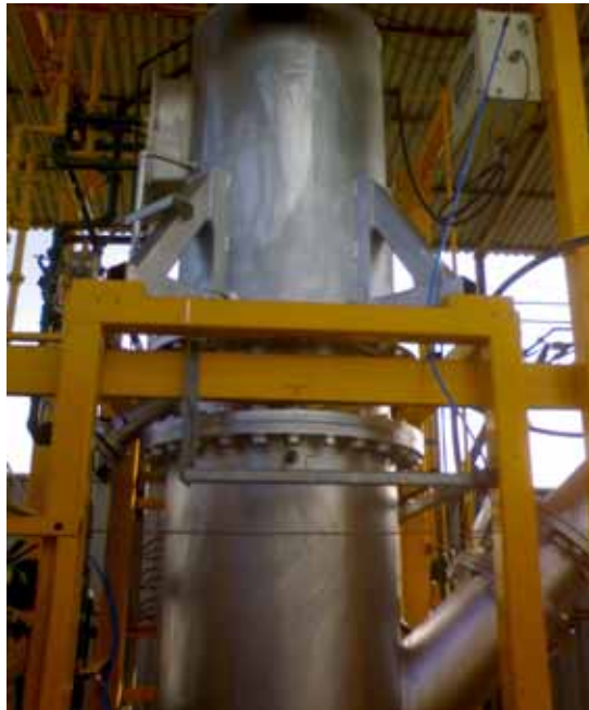
Photo 17. Secondary Combustion Chamber
