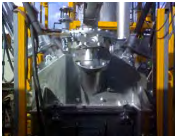
Photo 7. Gasification / vitrification furnace
